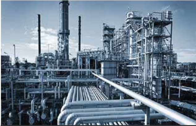
Endüstriyel Mekanik Tesisat Industrial Mechanical Installation
